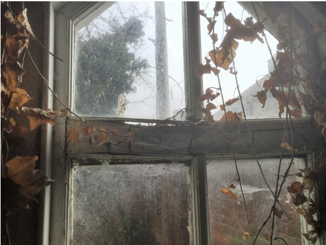
Vegetation growth within building and rot affecting window timbers internally
