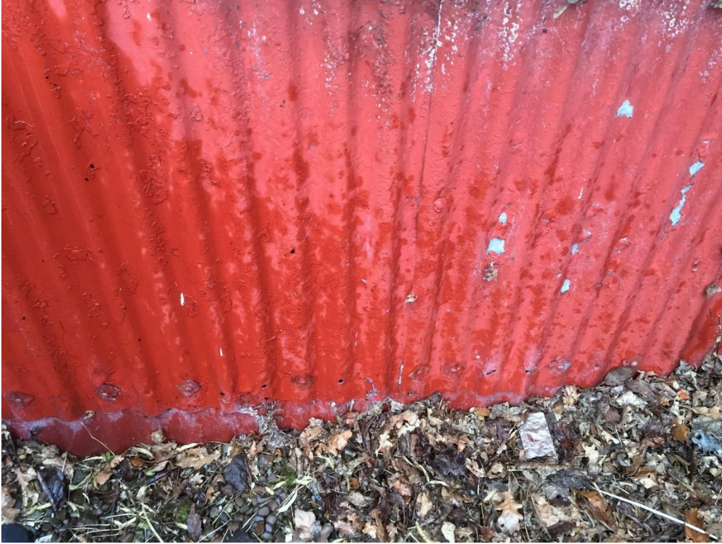
Holed and Corroded Metal Cladding
