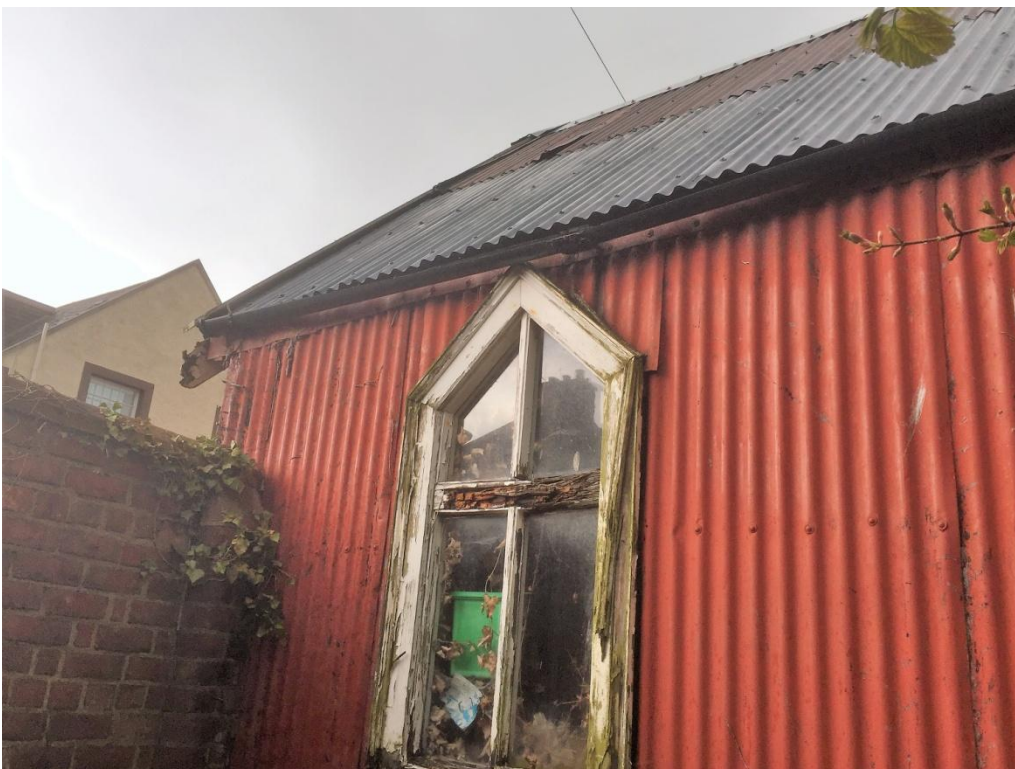
Rotted Window Timbers
