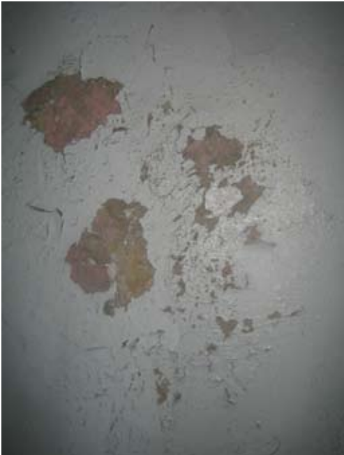
A modern, non-permeable emulsion paint flaking off lime plaster. ©Author
