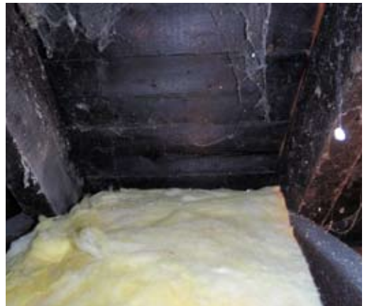
Fig 3. Mineral wool insulation can also be laid between rafters and joists, but with care not to inhibit air movement.
