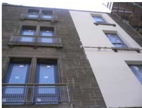
Fig 11. External insulation applied to an unlisted tenement has dramatically changed its architectural character.
